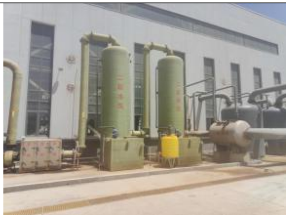
1#车间冷凝+二级碱洗+二级水洗+活性炭吸附
