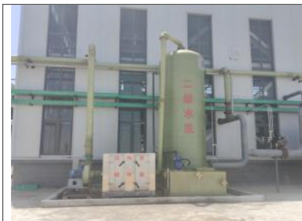
5#车间二级水洗+活性炭吸附
